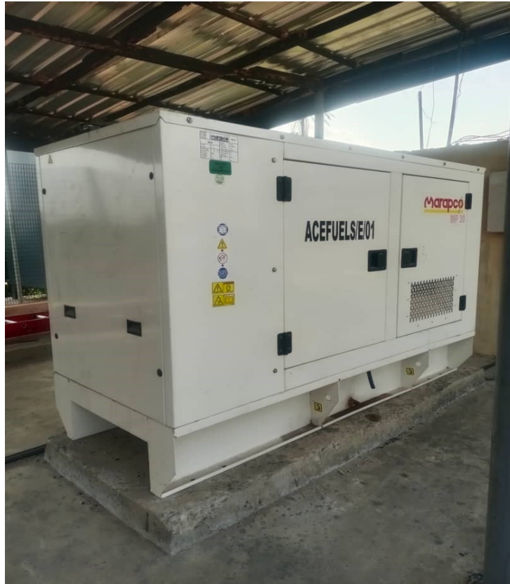
30KVA DIESEL GENERATOR
